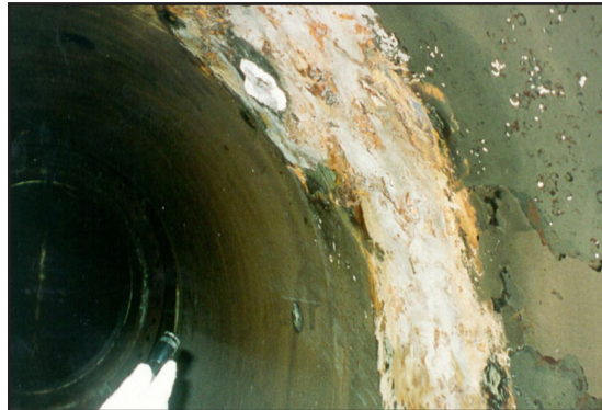
Significant corrosion in area of failed rubber lining
